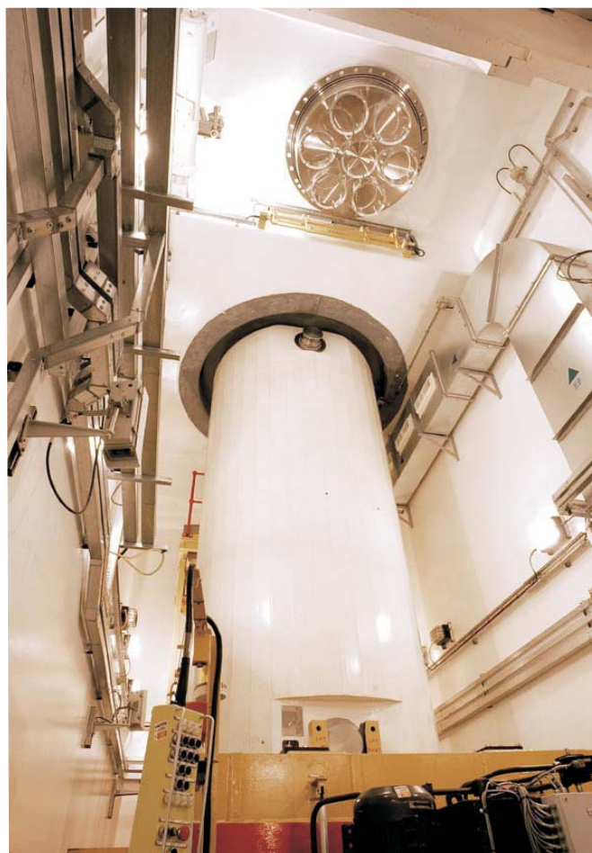
A VRR flask within the REF flasking cell where vitrified waste canisters are loaded into flasks
