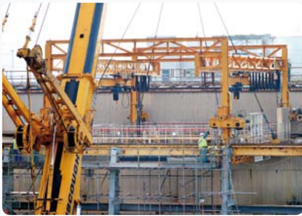
The Gantry Refurbishment System is lowered into place, a key enabler for future waste retrievals from the First Generation Magnox Storage Facility Pond
