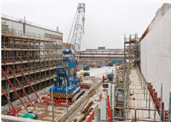
Construction of Sludge Packaging Plant 1, which will receive legacy sludge from the First Generation Magnox Storage Pond and process it into a product suitable for long term storage or disposal
