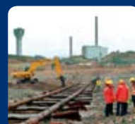
Sea discharge lines
