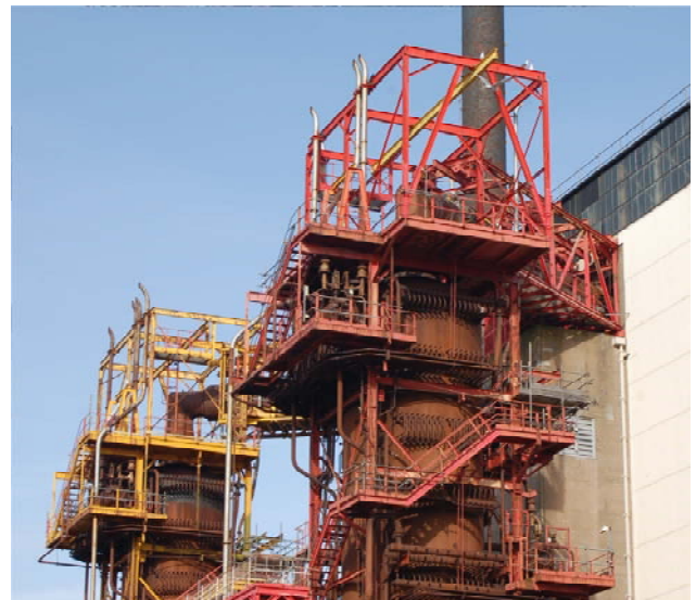
Calder Hall reactor four after the work was completed. The picture on page two shows the same scene before work began
